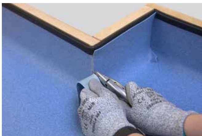
4. Carefully trim off all excess flooring, leaving a tightly fitted infill section.
