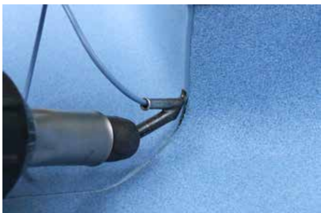
3. Weld the external mitre from top to bottom, being careful not to press the weldrod too firmly on the upstand section as this can cause damage to the flooring.
