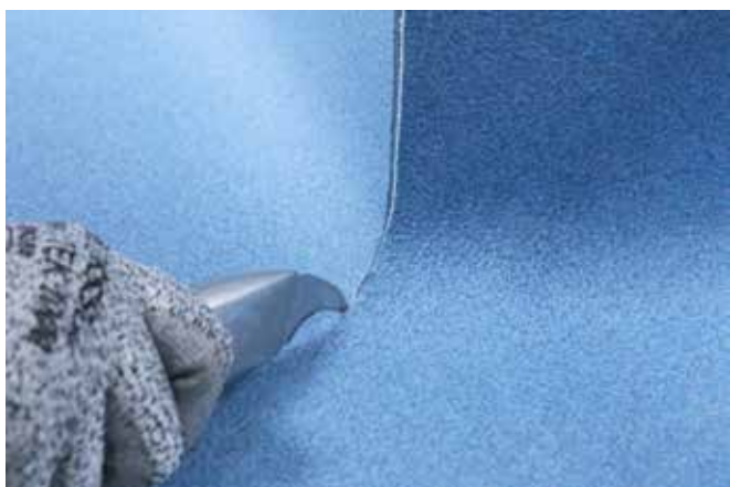
1. Use a concave blade to prepare the upstand and cove former sections, creating a 'V' section in preparation for hot welding.
