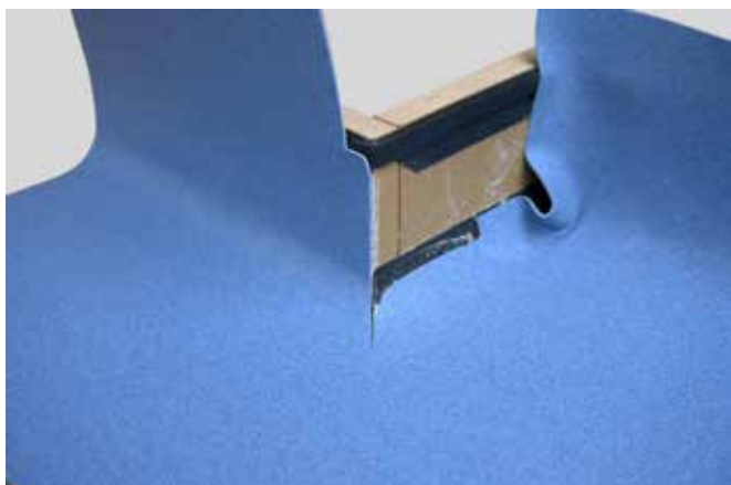
1. Fit the flooring to the closest/front wall. Cut down the external mitre, ensuring you have left sufficient excess to drop back into the internal mitre.
