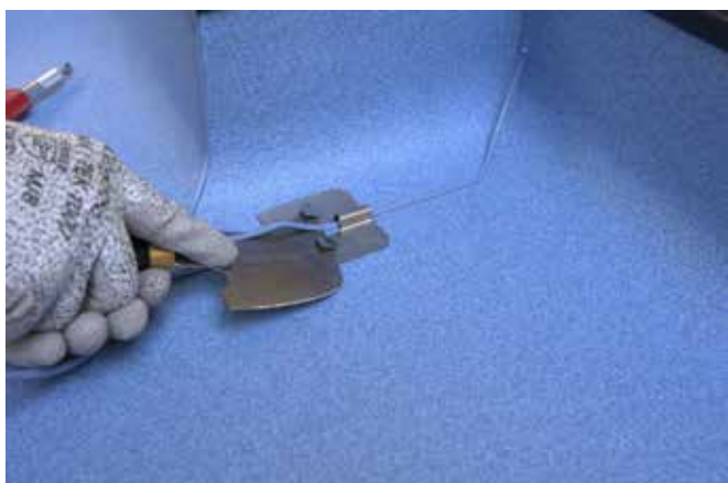
7. Allow the weldrod to cool completely, and trim off excess weld using sledge and spatula.
